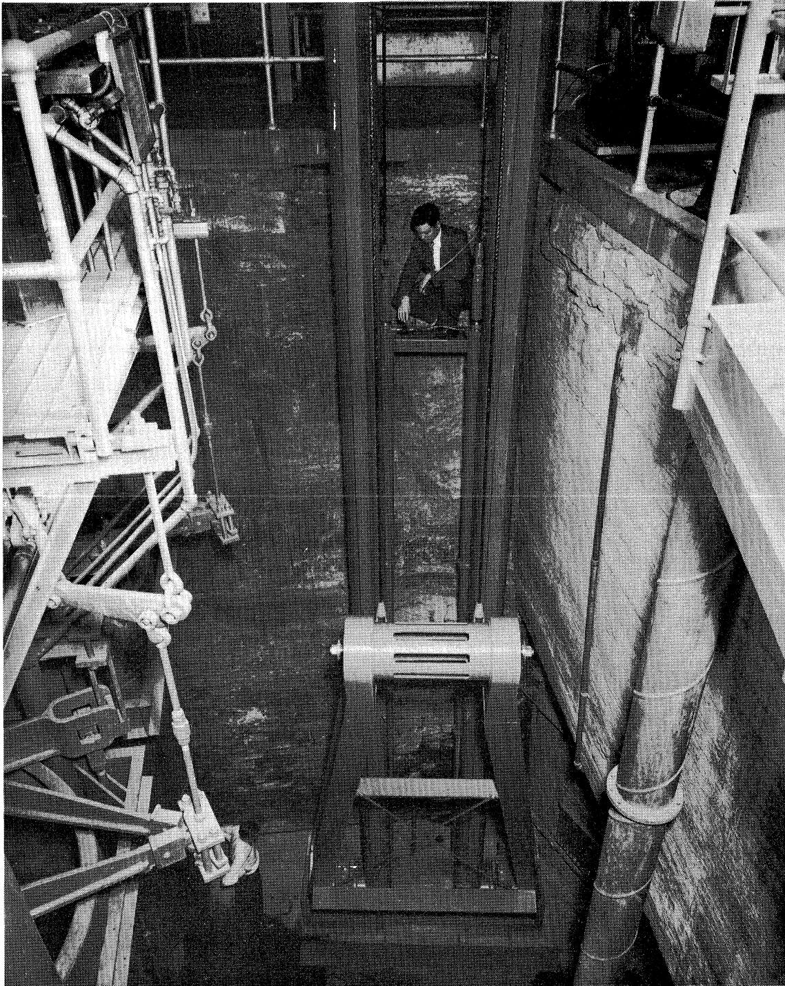
Fig. 8- Structure Before Attachment of Flume Spacer Cylinder in Place Between Monitor Arms
